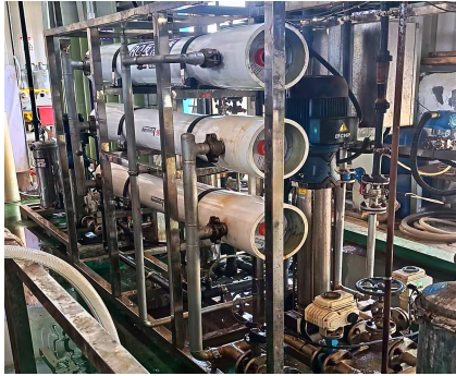
Reverse Osmosis System
