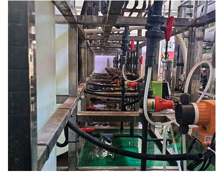
Chemical Dosing System
